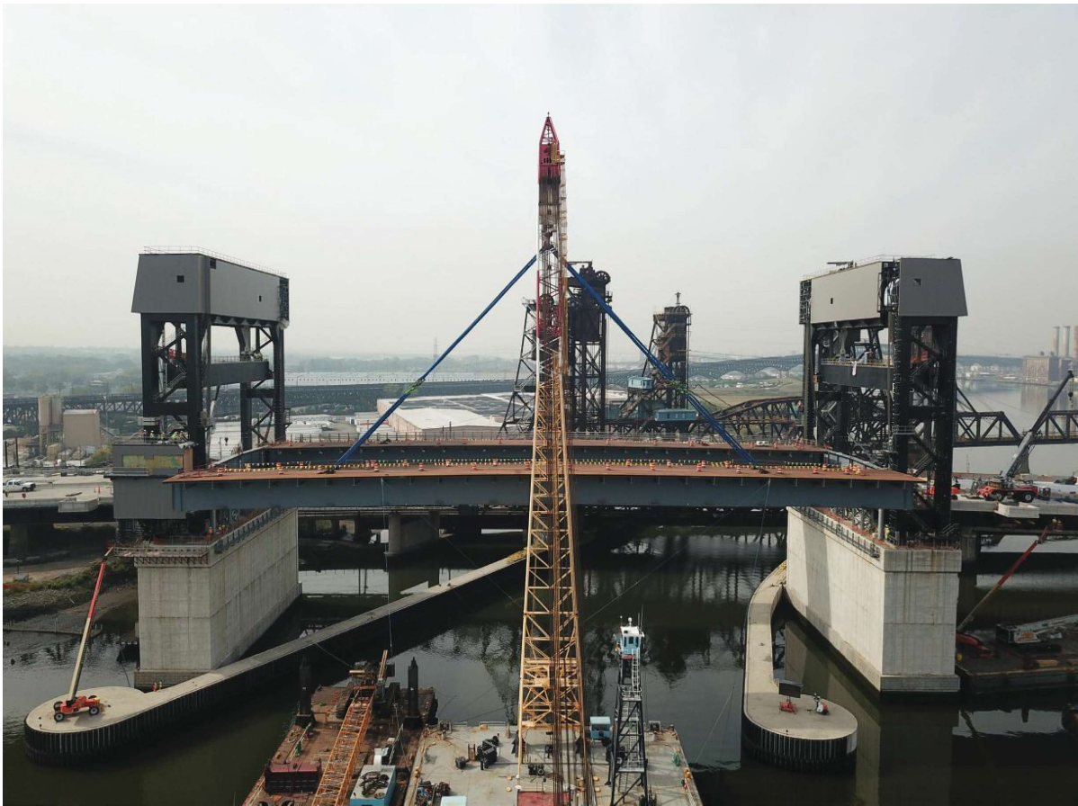
Three longitudinally split, approximately 700- ton deck spans were lifted into place, one per day. Courtesy of CCA Civil »
