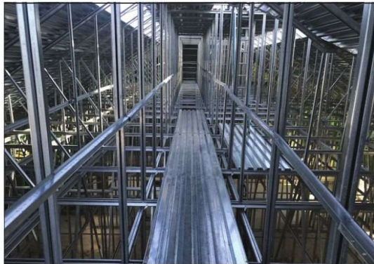
Light gauge steel trusses at Lakeside Park Place, a condominium development in Kingsville, Ont.
